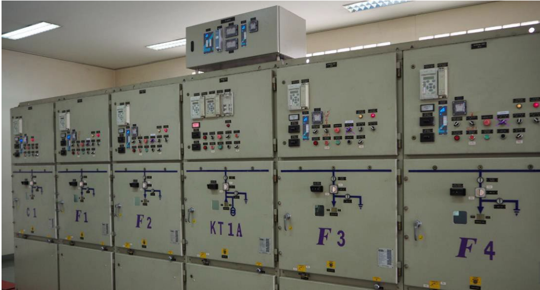
PEA EKA substation - arc protection
