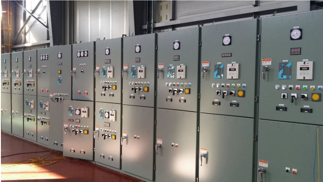
Pohang 3 Cokes switchgear
