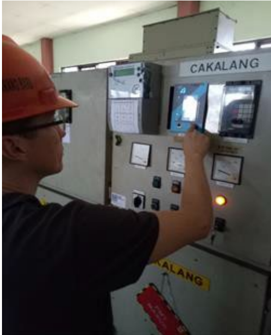
PLN Cakalang substation
