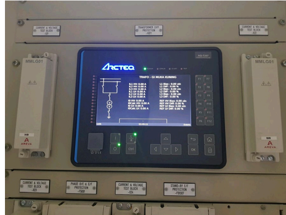
PLN Batam substation
