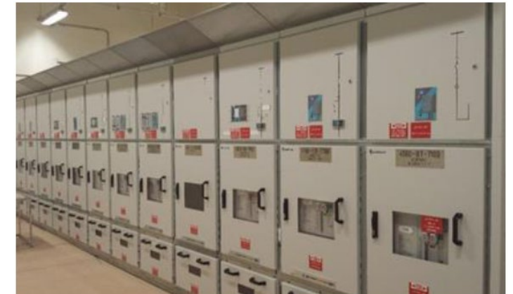
Arcteq supplied the Ma'aden Bauxite & Alumina Company with AQ-G357 and AQ-F215 type of generator and feeder protection
